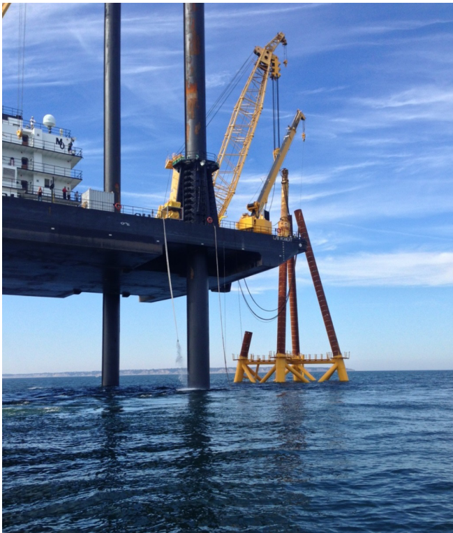
The 30-MW Block Island Wind Farm under construction. Photo courtesy of Deepwater Wind.
